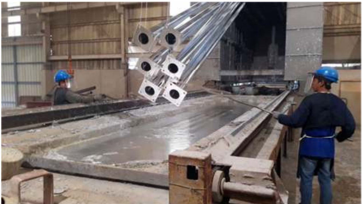
Preparing to hot dip galvanize a batch of steel tubes in a bath of molten zinc
